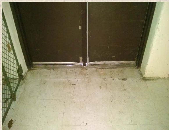
ALUMINUM ENTRANCE THRESHOLDS MISSING OR DAMAGED AT 4 ENTRANCES
