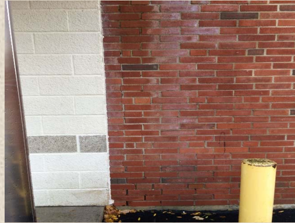
DETERIORATED BRICK/MORTAR JOINTS & SEALANT
