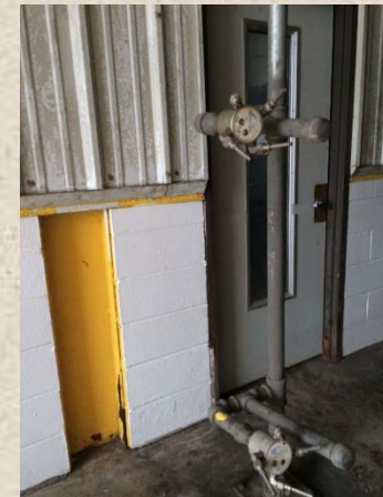
REPLACE DETERIORATED PANELS IN WASH BAY, RE-SECURE REMAINING
