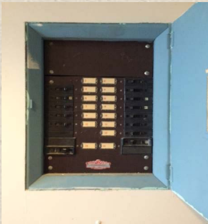
INTERIOR ELECTRICAL DISTRIBUTION
