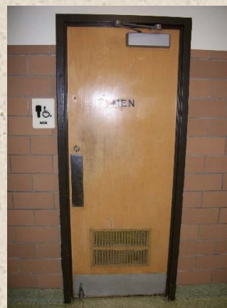
INTERIOR DOORS DETERIORATED & NON-RATED DOORS
