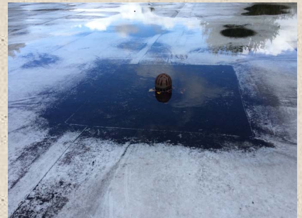
REPLACE ROOF DRAINS, IMPROVE DRAINAGE, ADD ADDITIONAL DRAINS
