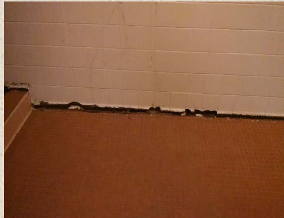
GYMNASIUM & LOCKER ROOM EXCESSIVE SETTLEMENT
