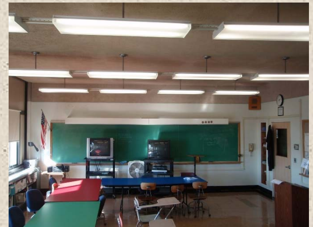
ACM PLASTER CEILINGS REMAIN IN PORTIONS OF ORIGINAL FACILITY
