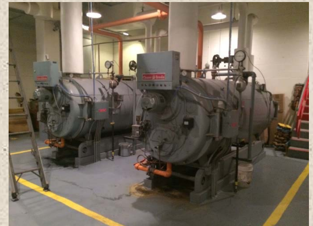
HEAT GENERATING SYSTEMS
