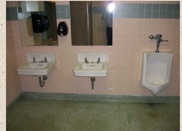
NON-AUTO, METERED FAUCETS PRESENT IN TOILET ROOMS
