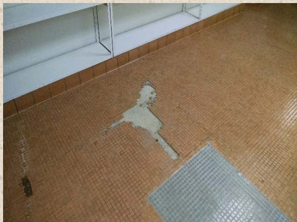
MAJORITY OF TILE IS VAT, SLAB IRREGULARITIES TELEGRAPH THROUGH ALL AREAS
