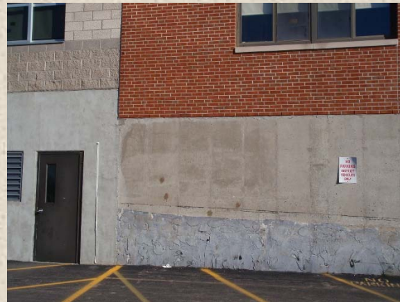
CONCRETE CORNERS AT FOUNDATION WALLS ARE SPALLED AND DETERIORATED.
