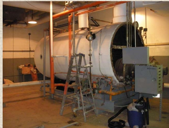
HEAT GENERATING SYSTEM
