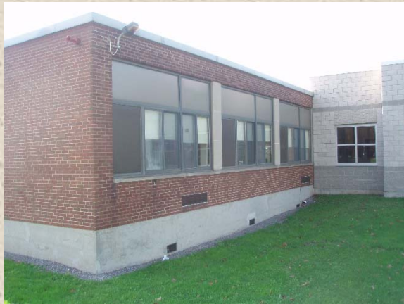
GROUND WATER INFILTRATION ALONG EAST WING NO OTHER DISCHARGE POINT
